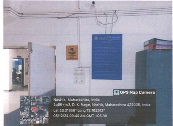
CCTV in Computer Lab
