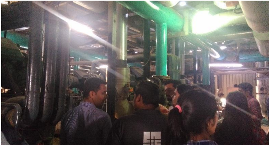
Plant room and air handling unit
