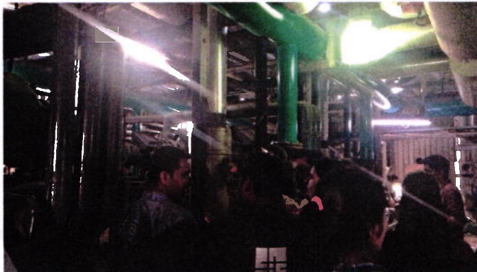
Plant room and air handling unit
