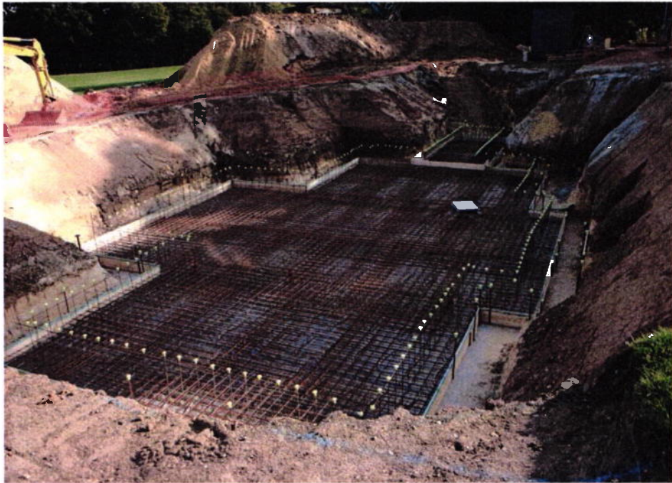
Box excavation done and reinforcement ready for raft slab ready at a construction site
